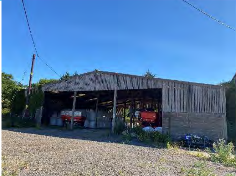
An open large agricultural building in use that was found to support a day roost used by two common pipistrelle bats (Confirmed roost)
